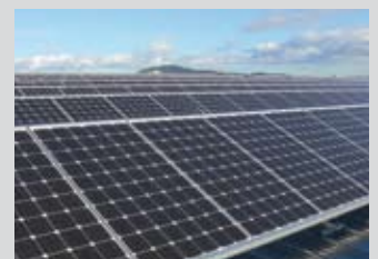
Gisinger Solarpark, Freiburg, 187 kWp
